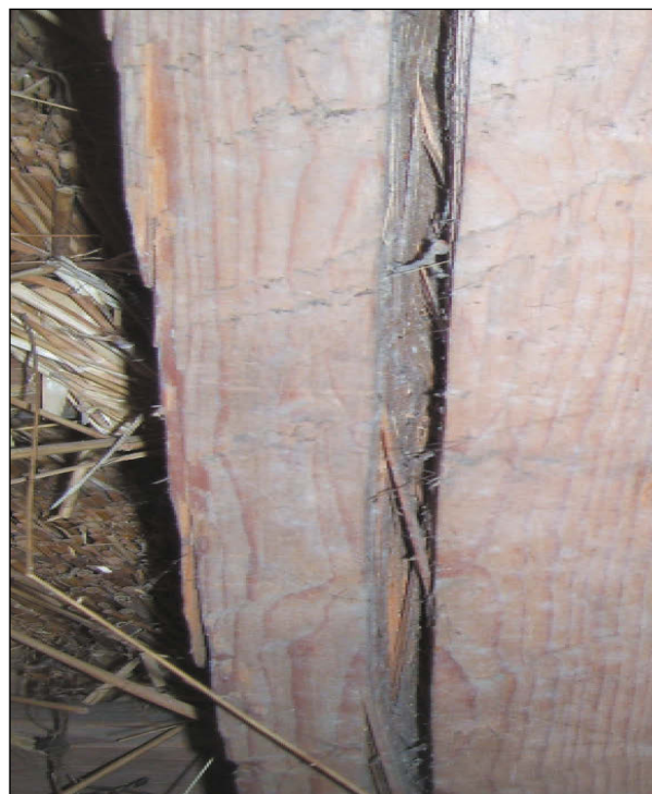
Fig. 4. Longitudinal rafter crack – cottage from Teodorówka.
