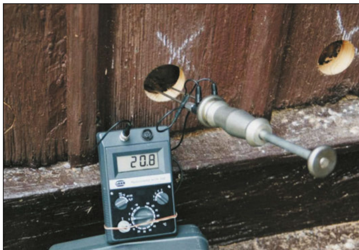
Fig. 1. The Church of Transfiguration in Żuków – using resistance hygrometer to measure the humidity of the foundation, (Fig. K. Krajewski).
