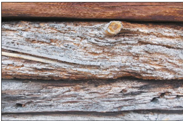
Fig. 5. Biological corrosion – cottage of Janiszowia.
