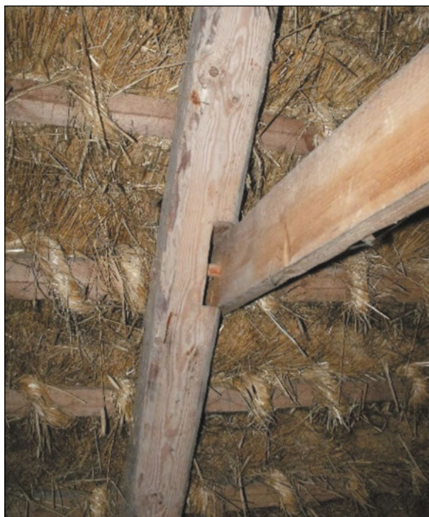
Fig. 3. Damaged joint between rafter and collar beam – cottage from Żabno.
