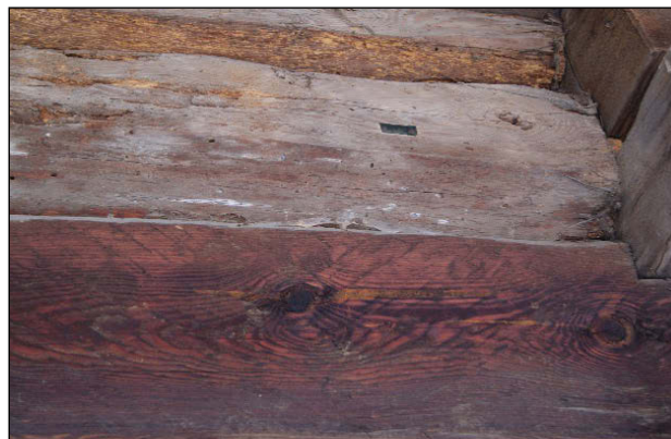
Fig. 6. Biological corrosion and the state of wood treatment – cottage of Brzeziny.
