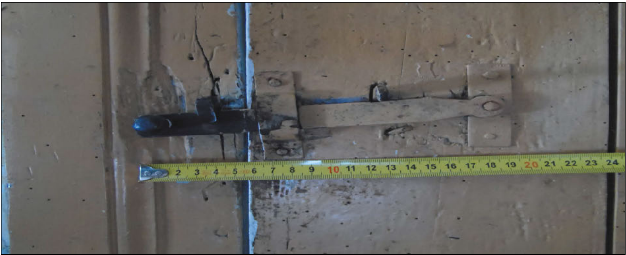
Fig. 3. Cottage in Tymianki Moderki. Door lock detail, digital photography with tape measure, 2013.
