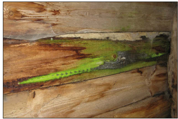
Fig. 8. Result of excessive moisture on walls – circular Urzędowo.
