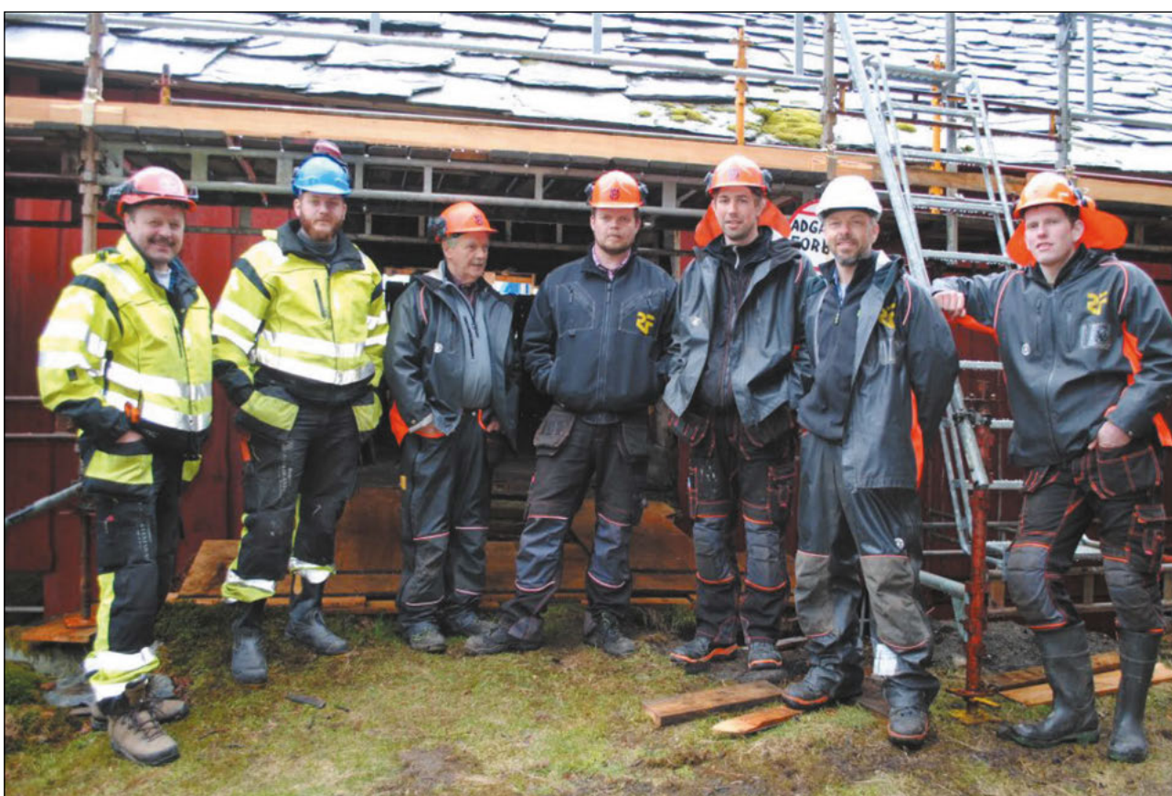
Fig. 3. During restoration work on Viga farm we were able to use three permanent employees and two project craftsmen in addition to two more who were hired to help with technical solutions. Planning and management were done by the head of the Buildings Department (not present in the photo).
